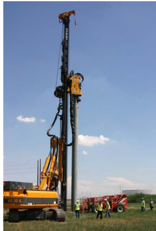
A low-amplitude vibratory pile driver sinks each pedestal 18 feet into the ground. No excavation is required, no grading is necessary and no concrete is poured. This will make remediation simple and fast when, decades in the future, it is time to decommission.
